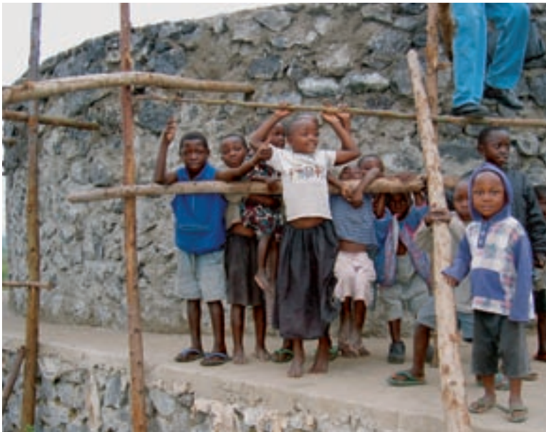
Anticipation and curiosity: children follow the progress of the construction of the reservoir in Mugunga.
