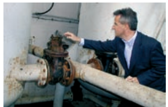
Rolf Leutert, Managing Director of the “Clean Water” Foundation from 2002 to 2005, visiting the project site in Dobrich. These pipes no longer serve their purpose.
